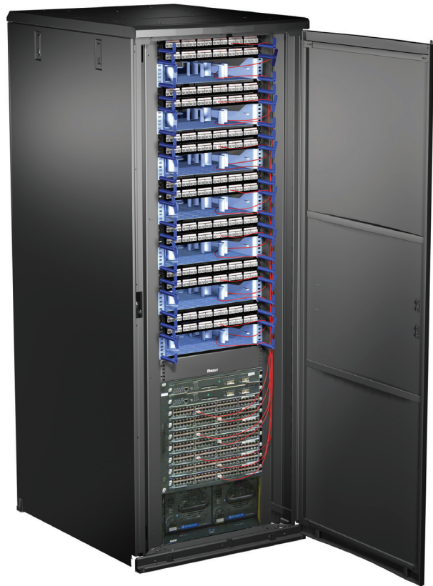
Figure 2: Application of a horizontal slack manager and bend radius posts installed in a full size cabinet
