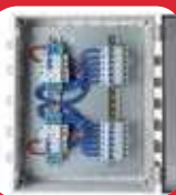
9. DC surge protection
