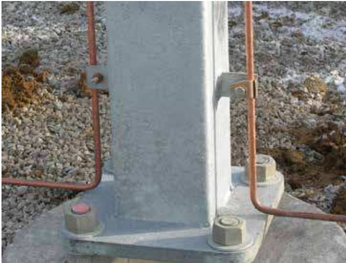
Substation earthing riser
