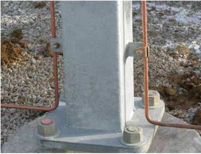
Substation earthing riser
