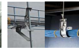
Cables from threaded rod
