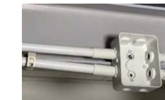
Conduits & electric box from beam
