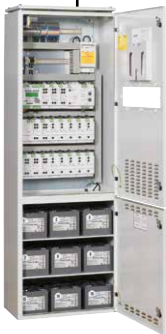
CEAG emergency lighting supply unit (non-hazardous area)
