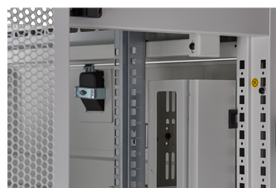
High-density vertical cable management
