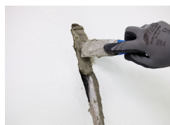
Close the damaged area discreetly.
